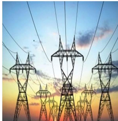
Electricity Transmission Lines
