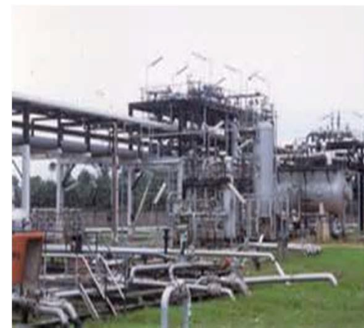
Nigeria gas production facility ( sweetcrudereports.com )
